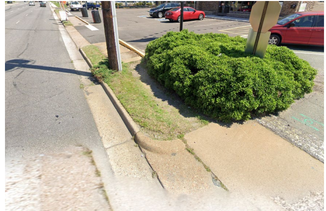
Figure 25. Poor Sidewalk Conditions and ADA Accessibility on Staples Mill Road near the Dumbarton Square Shopping Center
