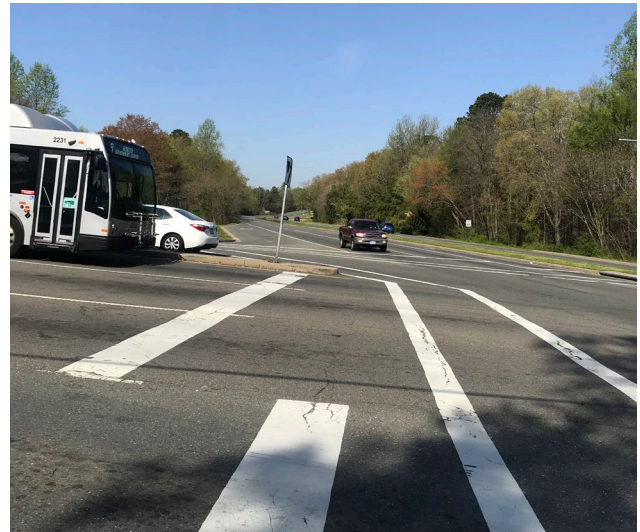
Figure 23. Skewed Crosswalk at E. Parham Road and Hungary Spring Road
