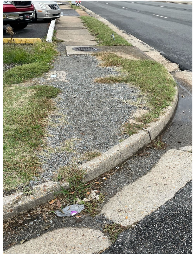
Figure 35. Substandard Sidewalk with Loose Gravel
