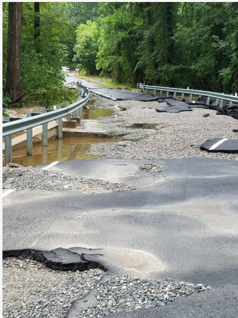
Figure 1: Emergency repairs will be needed prior to reopening Route 634 (Highgate Road) in Surry County.
