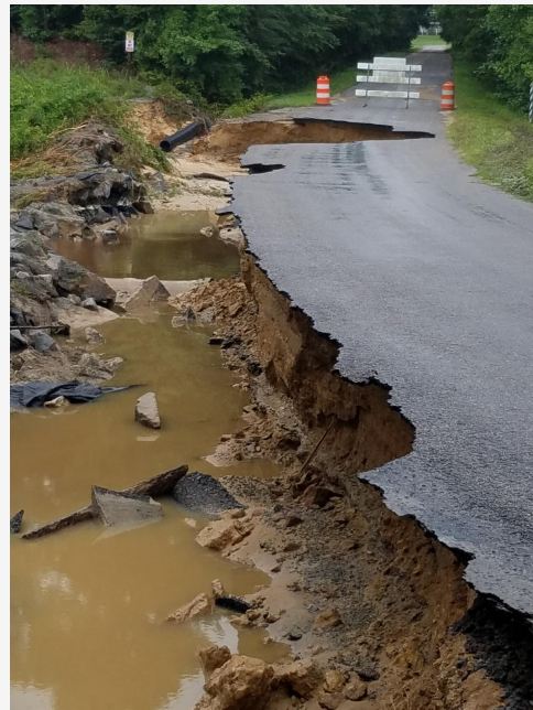
Figure 2: Washout damage to Route 650 (Mounts Ray Road) in Surry County.
