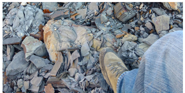
Above Photo: This region is known to be underlain by shale formations that tend to weather rapidly once excavated, which could be problematic if not identified.
