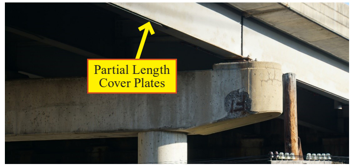
Above Photos: Looking west along Augusta Woods Drive below I-81 SB, showing BBRR ROW to the right and the existing retaining wall structure to the left ( top ). The pier on this bridges provides an example of substructure condition, configuration, and partial length cover plates ( bottom ).
