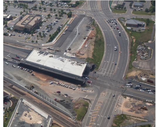
Figure 2 - US 29/Linton Hall Road Diversions where all movements were maintained with a signalized intersection adjacent to bridge and ramp construction.
